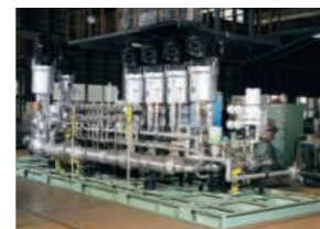
▲ Fuel gas flow control unit
