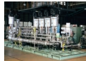
▲ Fuel gas flow control unit
